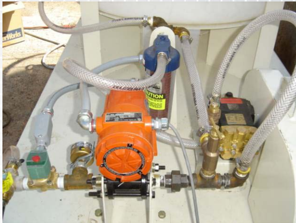
Water system detail
