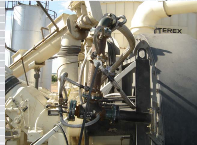
Mixing chamber and piping installed (no insulation)
