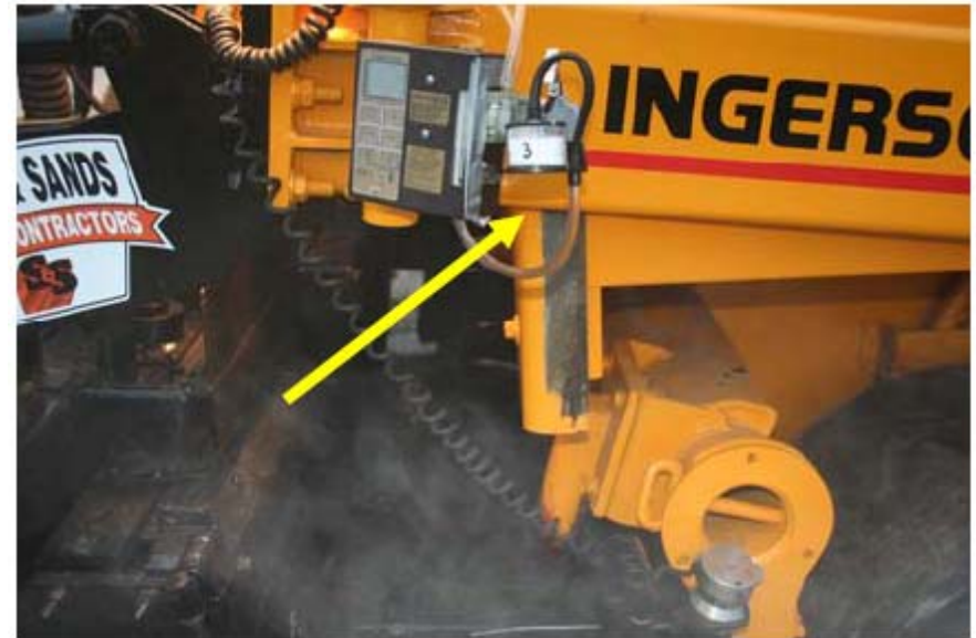
Sample Location 3 – Right Side Screed Discharge over Auger
