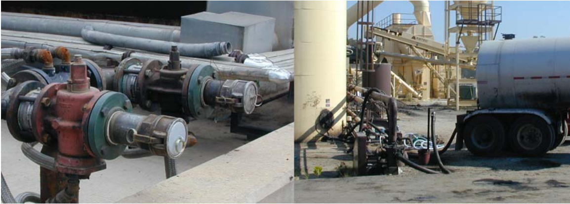
Figure 1. a) Heated Valves Allowing Recirculation and b) Tanker Pumping Evotherm Directly into Plant.
